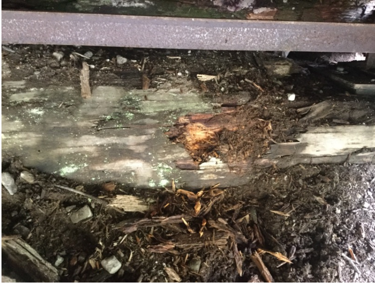
Log sill condition
