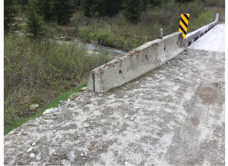
Missing bull nose at upstream right bank
